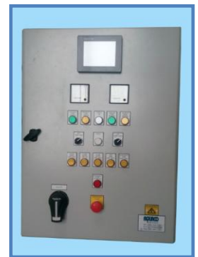
MBR control panel
